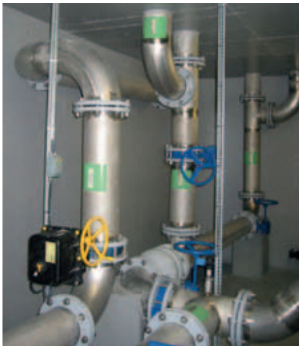
Figur 7.1: Ventilkammer under basseng
