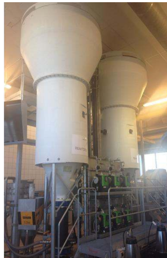
Figure 1 - Struvite reactors, Aaby WWTP
